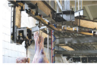
TRANSFERRING STATION Hydraulic transfer equipment is located in this section. The cattle is transferred from the bleeding line to the processing line.
